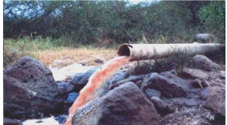
Figure 2. Free discharge of raw wastewater
